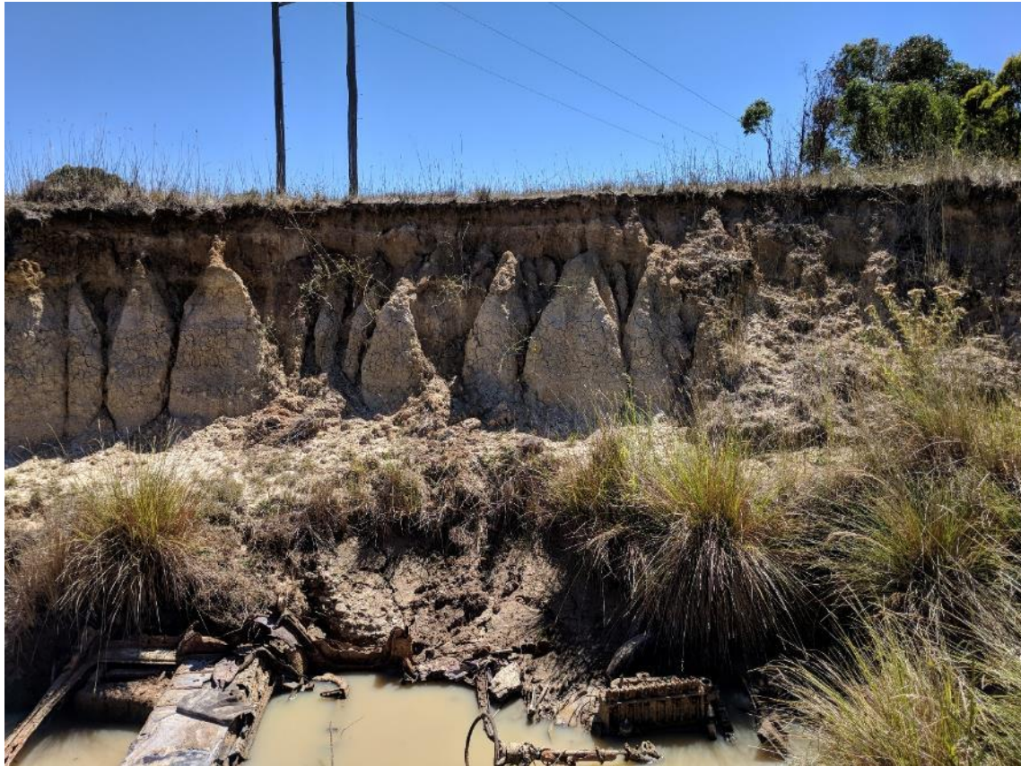
Figure 6-1: Example 1 of erosion within Church Creek
