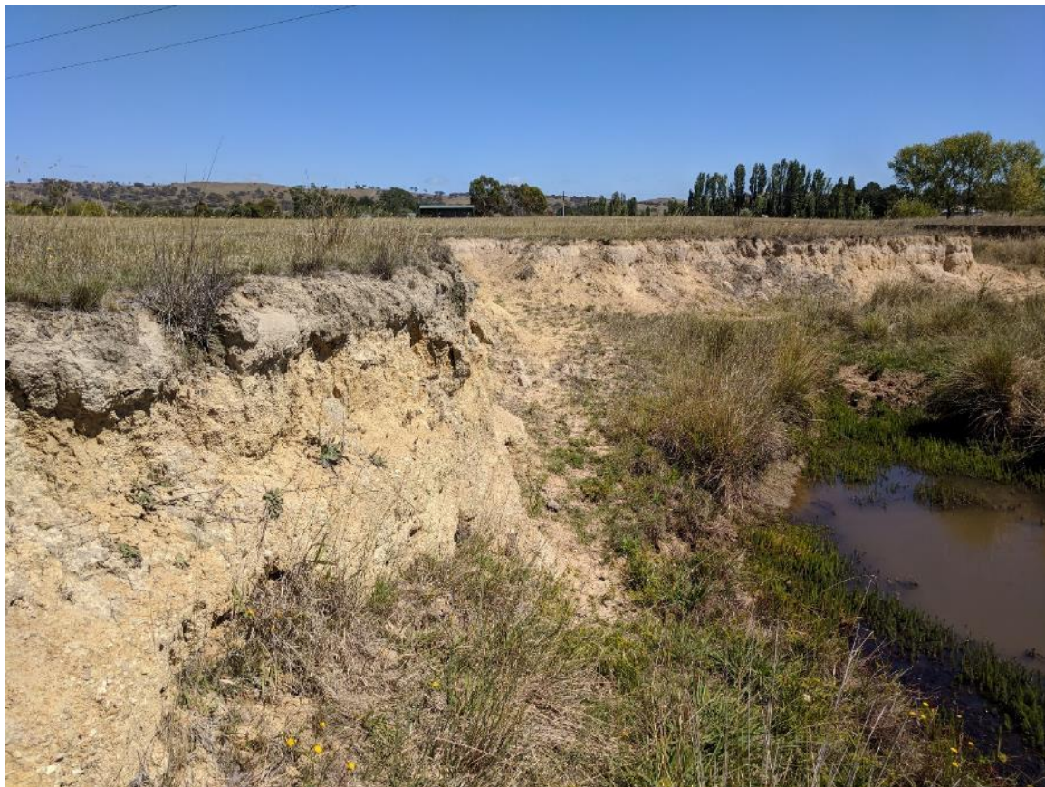
Figure 6-2: Example 2 of erosion within Church Creek
